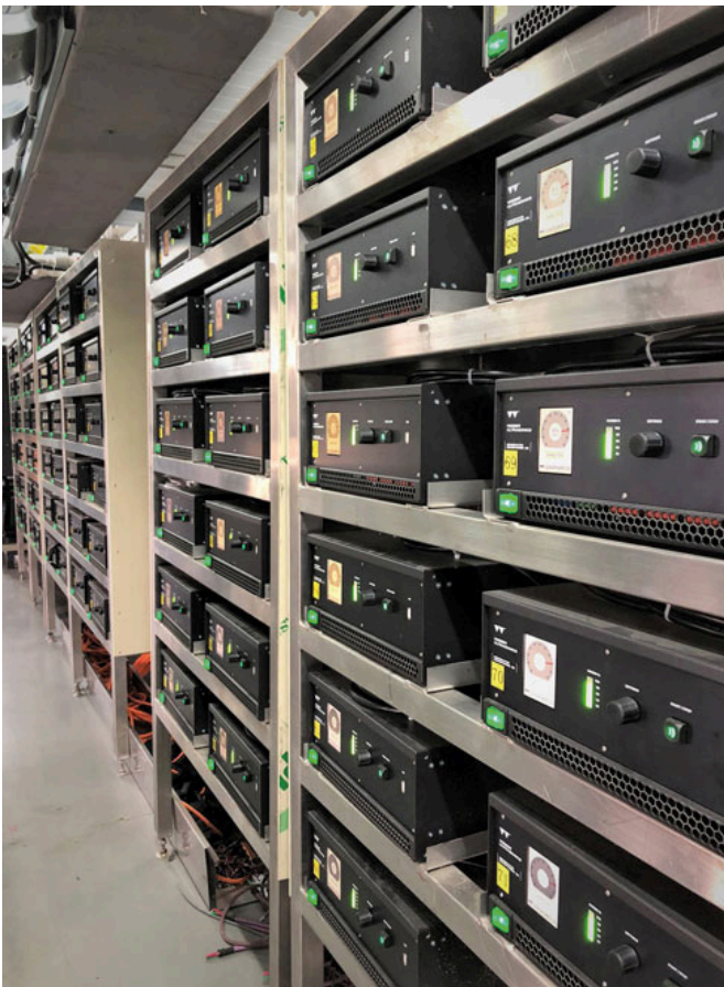
The 72 Sonopower 3S generators are located in an air-conditioned room and are equipped with an optional Profibus interface. This enables the transducers to be controlled remotely. (Image source: Weber Ultrasonics AG)
