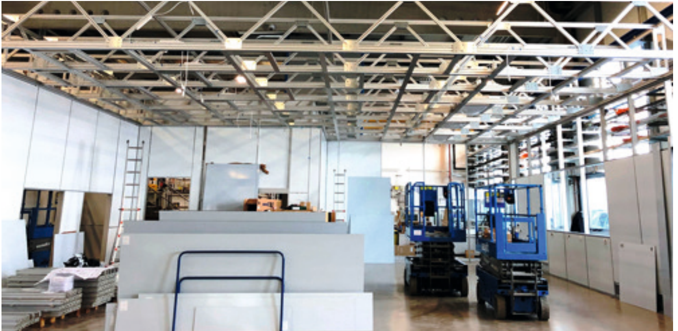
Since no suspension was possible on the on-site ceiling, the cleanroom was designed to be self-supporting using a truss made of aluminum profiles.
