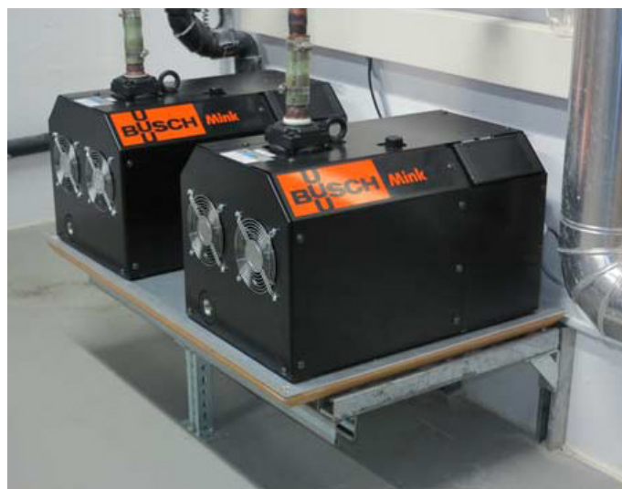
Fig. 1: Two redundant Mink MV claw vacuum pumps from Busch in the engineering room of the laboratory centre.
