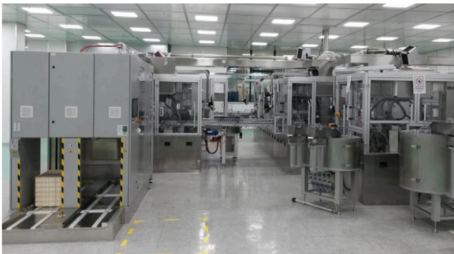
Hall 2 (assembly line) at Gerresheimer Regensburg GmbH in Pfreimd has been fitted with more powerful, more energy-efficient technology.
