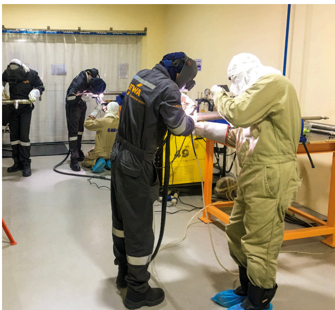
The material used for piping is titanium material (Grade 2), in total 58 meters of pipe ranging from ½ to 2 inches diameter with 339 welded joints have been completed. To meet the stringent requirements for welding joint quality, LEWA NIKKISO Middle East built its own clean room. (Source: LEWA NIKKISO Middle East FZE)
