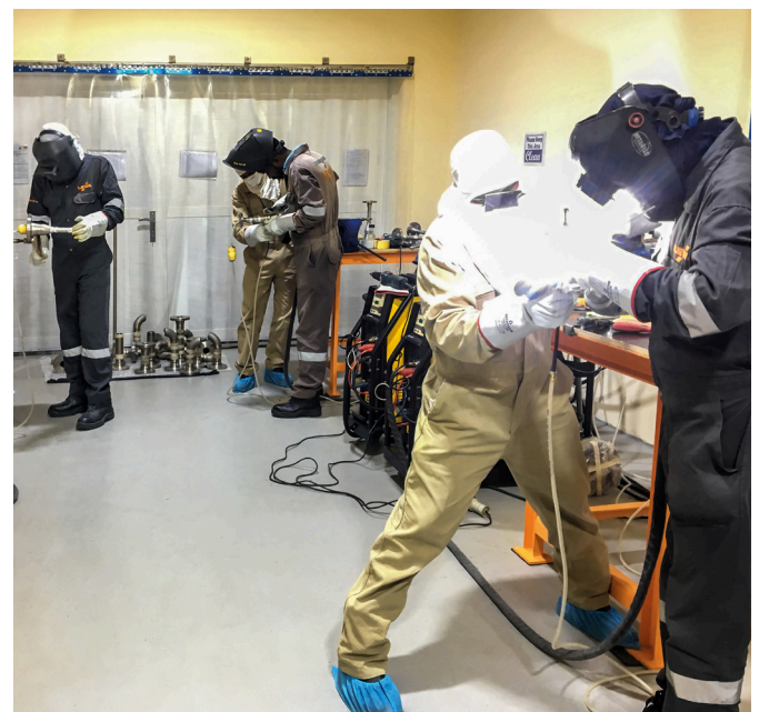
During welding, an auxiliary welder held the shield diffuser, ensuring optimum coverage of the heat-affected zones with pure argon gas. (Source: LEWA NIKKISO Middle East FZE)
