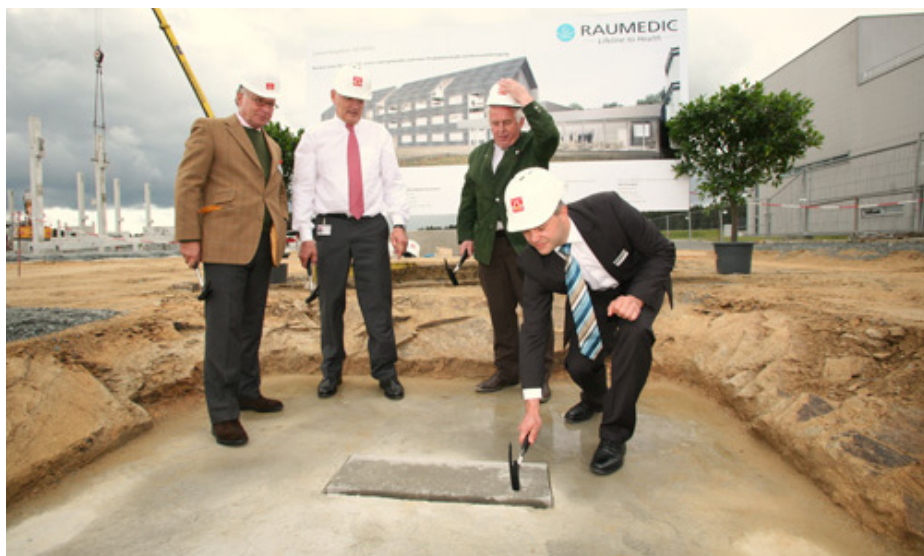
Best wishes for a good construction project and a continued business growth with symbolic hammer blows (from left): Jobst Wagner, President of the REHAU Group, Martin Bayer, CEO of RAUMEDIC AG, building contractor Alois Dechant and RAUMEDIC project leader Martin Silbermann (picture: Michael Giegold)
