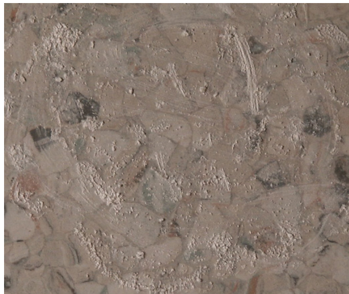
Image 4 (disinfectant residue on vinyl flooring)
