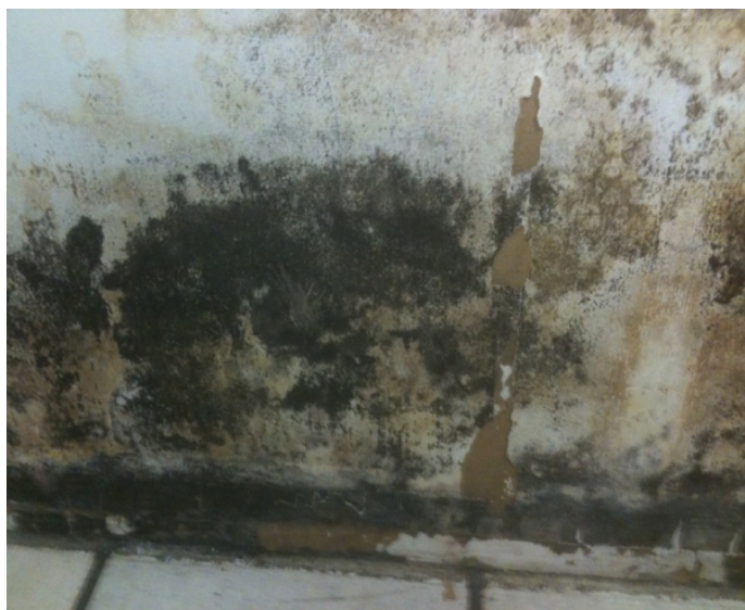
Image 1: Water damaged wall covered with mold. (photo by Jim Polarine)
