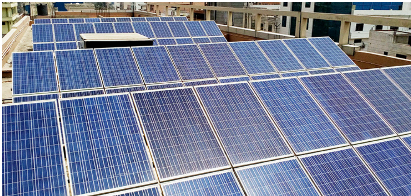
Solar panels on the roof of the Gerresheimer Triveni plant.
